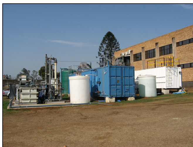
Figure 4.53 Three different Membrane Bio-Reactor Pilot Plants undergoing testing at Darvill WWWW.
