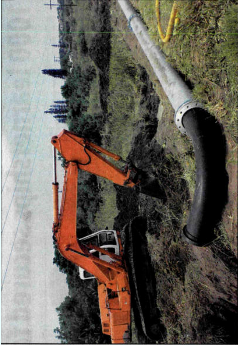
Contractors are seen using earthmoving equipment to repair the burst water pipe situated in a river in Grootville
